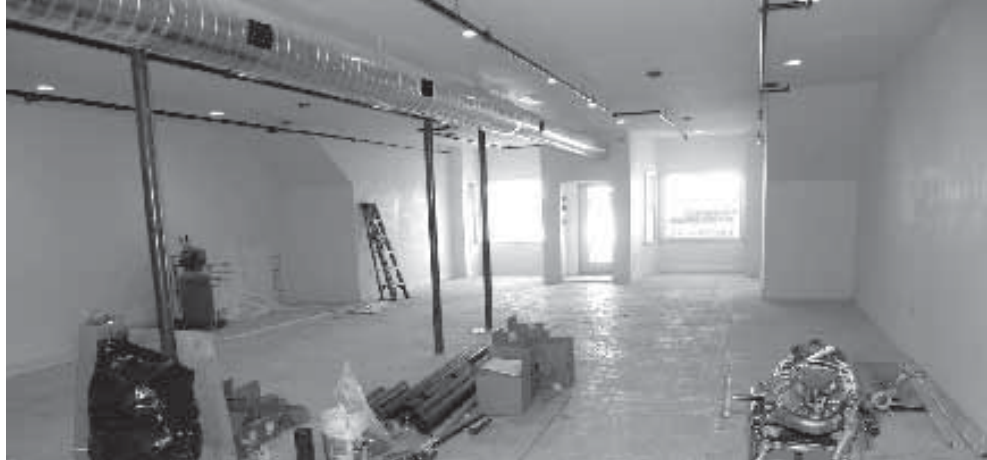
The interior of Buckley's Irish Pub remains barren as the building's owner waits for the certificate of occupancy.
