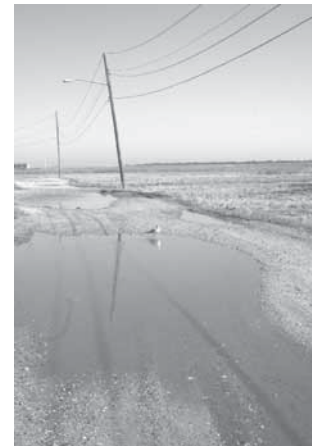
Drainage issues along Riviera Drive near Marina 5 in Mastic Beach has some residents concerned about the health of the wetlands. ADV/Hoey
